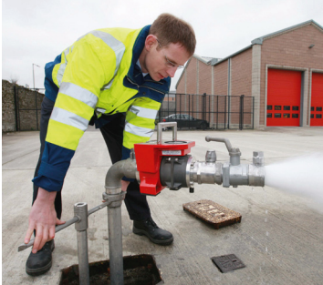
Fig. 1.2 Testing an underground fire hydrant
