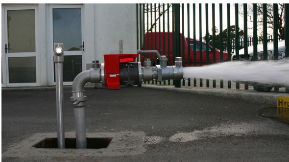
Fig. 4.3 Flow testing with ball valve to facilitate static and residual pressure measurements at Portlaoise Hospital. Photograph courtesy of Portlaoise Hospital Service
