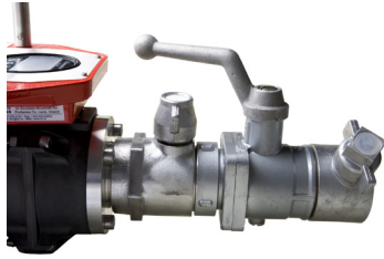
Fig. 7.1 Ball Valve to facilitate static pressure measurements
